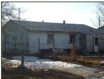
Abandoned homes with lead and asbestos contamination
